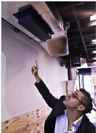
Fred R. Conrad/The New York Times Mr. Giordano describing a new ventilation system.
